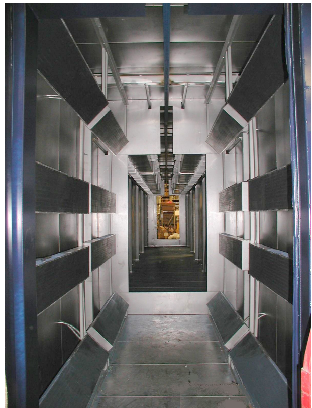
Typical Industrial Convection Oven.
